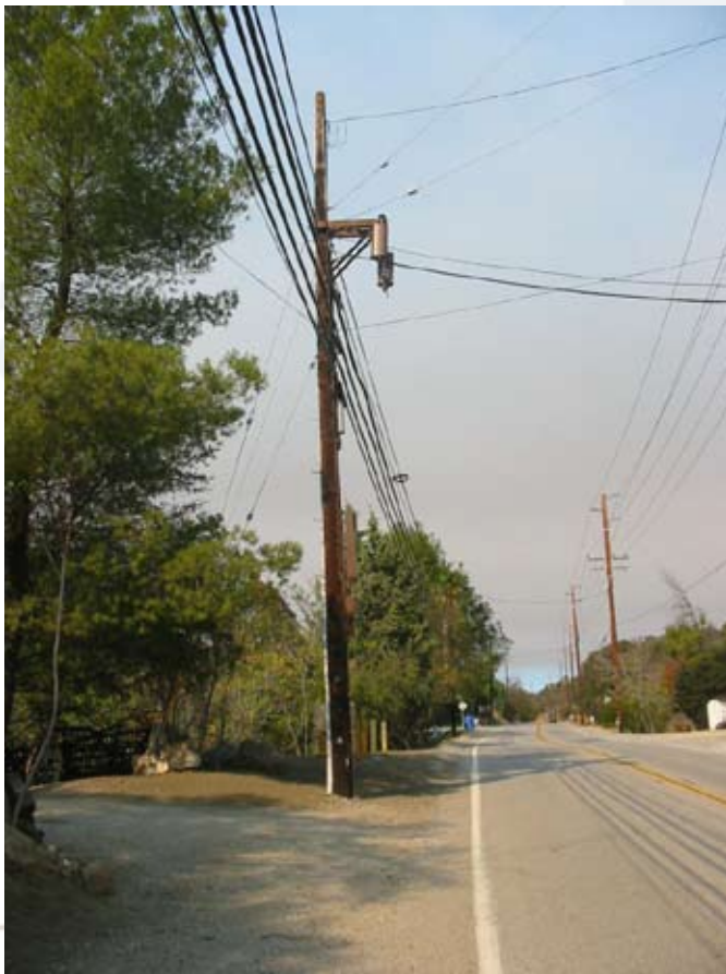
Example of utility pole mounted cell site
