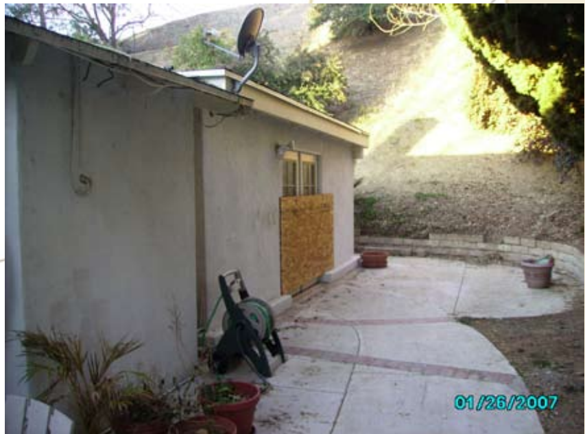
View of the illegal room addition
