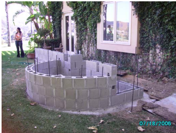
Un-permitted exterior structure (BBQ Grill), violation of the Los Angeles County Building Code & Zoning Code.
