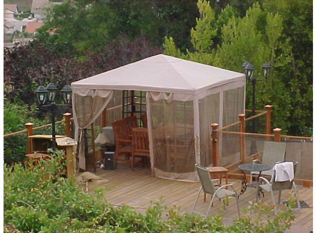
Un-permitted exterior deck/gazebo/lighting encroaching on property lines. Violation of the LACBC, Development Code and Municipal Code.
