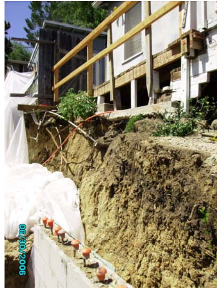
Illegally cut slope causing a danger to the neighboring property.
