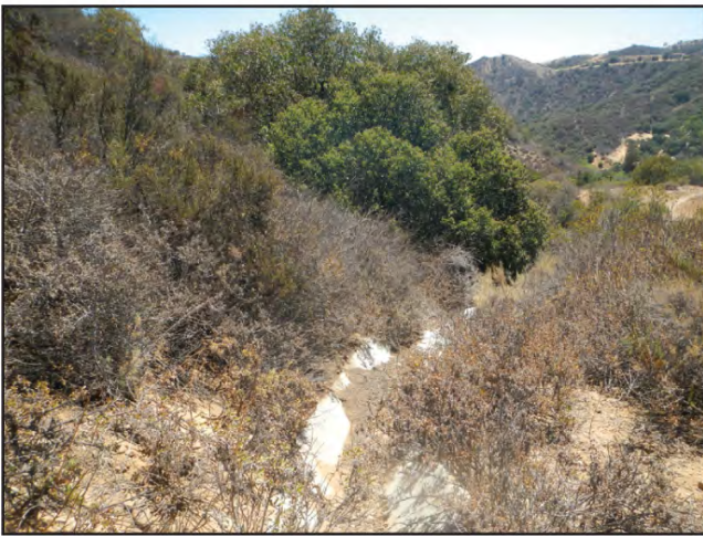
Photo 1C – View facing east of chamise and laurel sumac scrub surrounding a section of the concrete v-ditch to be repaired as part of the project.
