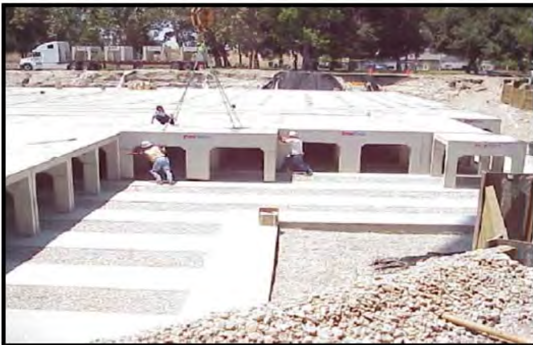
Sample Infiltration Gallery
