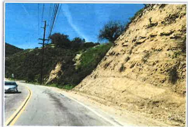
Michael Baker will assess various locations for possible retaining walls to reduce debris that flows into the street during rainstorms.
