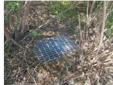
FIGURE 4.2.2.1b Grate inlet in Aster Tr.
