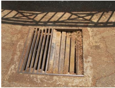
FIGURE 4.2.2.1a Grate inlet in Ivy Tr.
