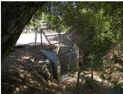
Figure 5.2.5a Inlet Facility with Debris Rack
