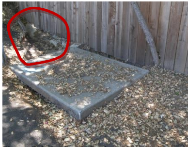
Figure 5.2.1a Catch Basin at Locust Dr.
