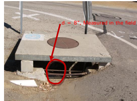
Figure 4.2.2.2b 4-Side Opening Inlet in Canyon Dr.
