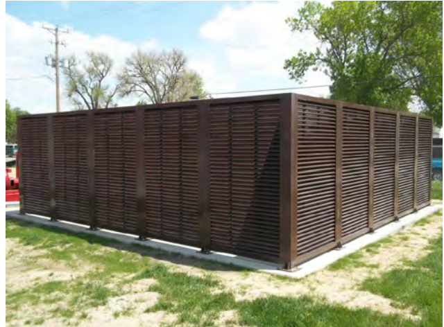
Figure 54: When transformers are infeasible to place underground, they shall be screened from public view with landscaping or walls. (Section 6.2.1)
