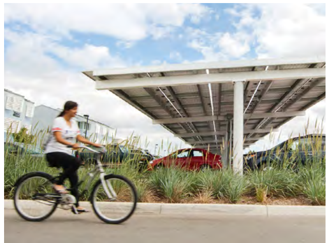
Figure 55: Ground-mounted solar equipment is located outside of setback requirements or required open space areas and does not obstruct travel. (Section 6.2.2)
