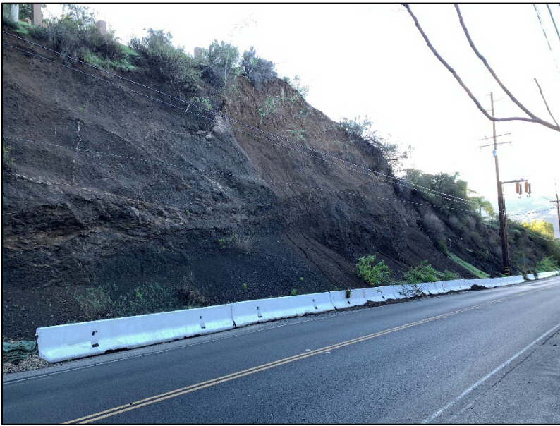
a. Slope to be stabilized with pinned shotcrete near Turtle Creek Road
