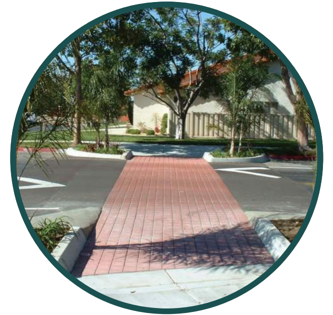
Raised Crossings & Intersections
