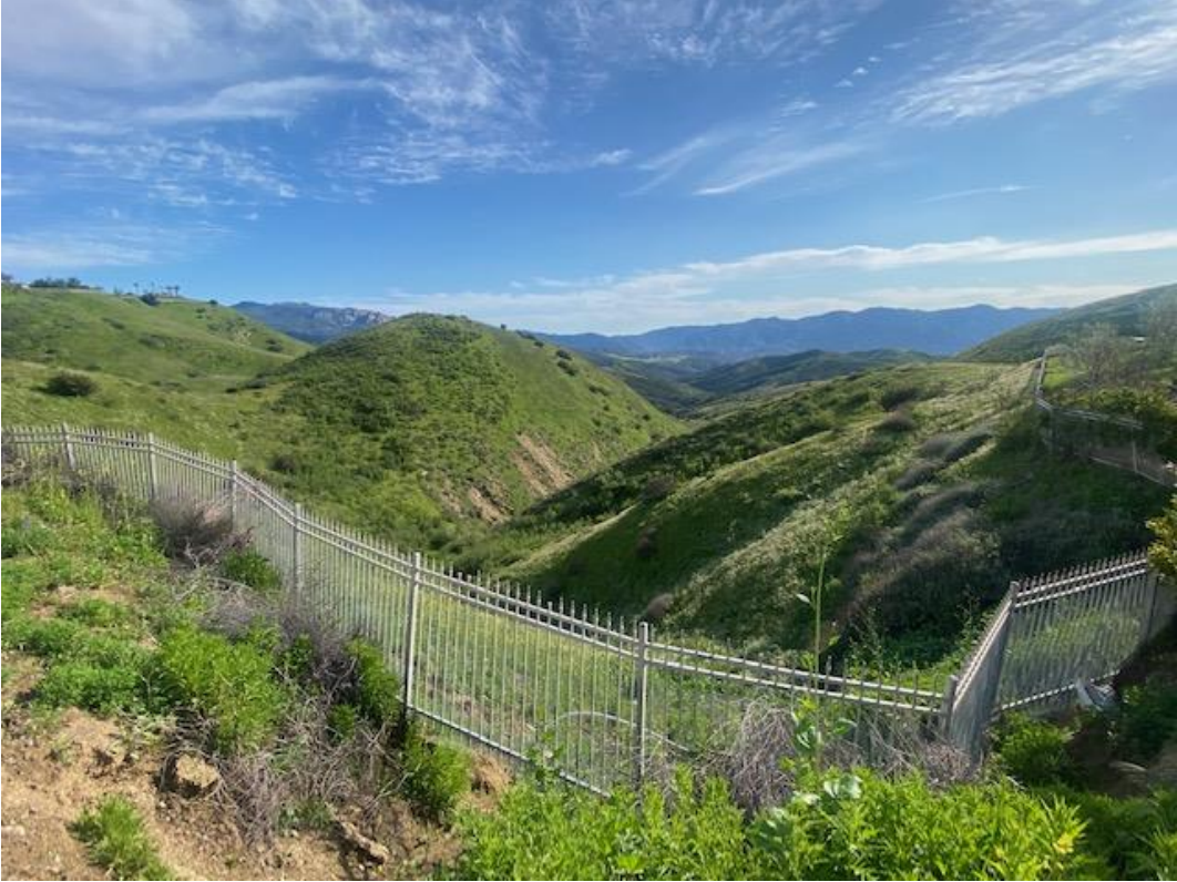
Photos 5-8: Taken after recent rains, exposed footings now covered by grass
