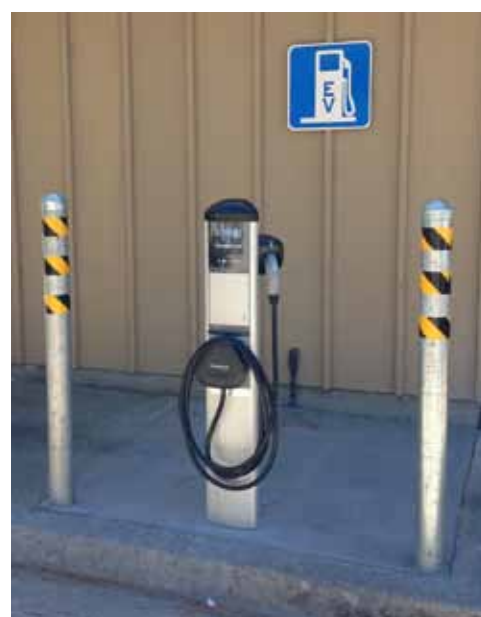
Electric vehicle charging station near Hauke Park
