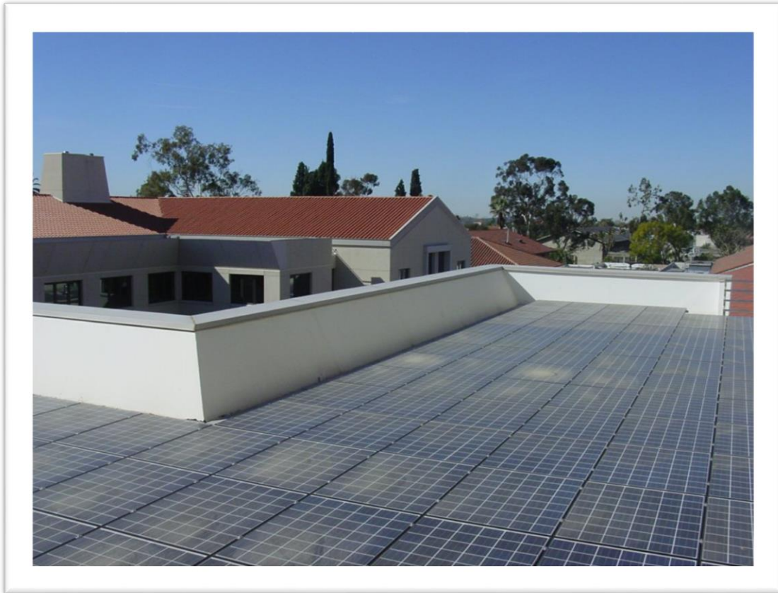
Figure 12 - Solar electric panels: Pomona College Science Building
