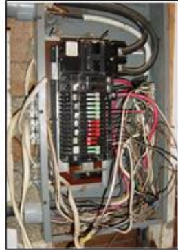
*Poor wire management
