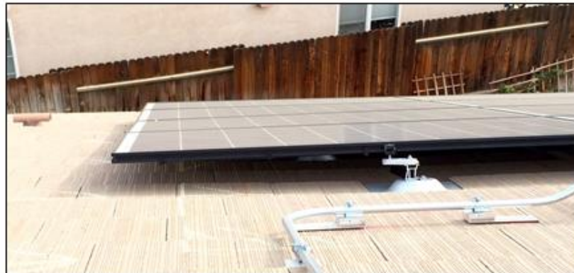
“Before” – Maximum cantilever of rack system exceeded
