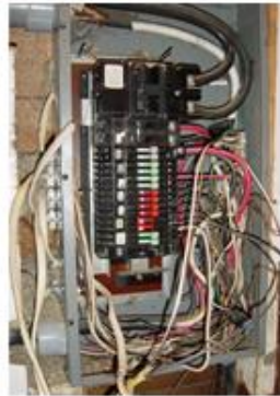
*Poor wire management
