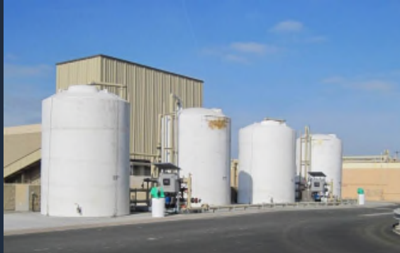
LA County Sanitation Districts, Carson, California (food waste slurry receiving tanks)
