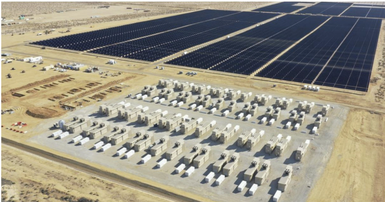
In November 2021, CPA began receiving 100 MW of clean energy storage capacity from Terra-Gen's Edwards Sanborn Solar-plus-Storage facility.
