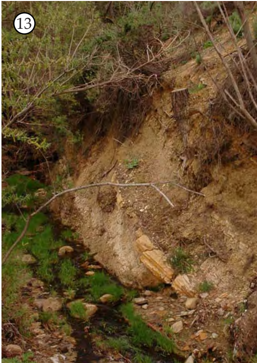
13 Dry Canyon Creek's channel was relocated to the base of a steep slope in the early 1950s. This straightened the stream and also shortened its length. The slope is bare and at risk of eroding into the stream.
