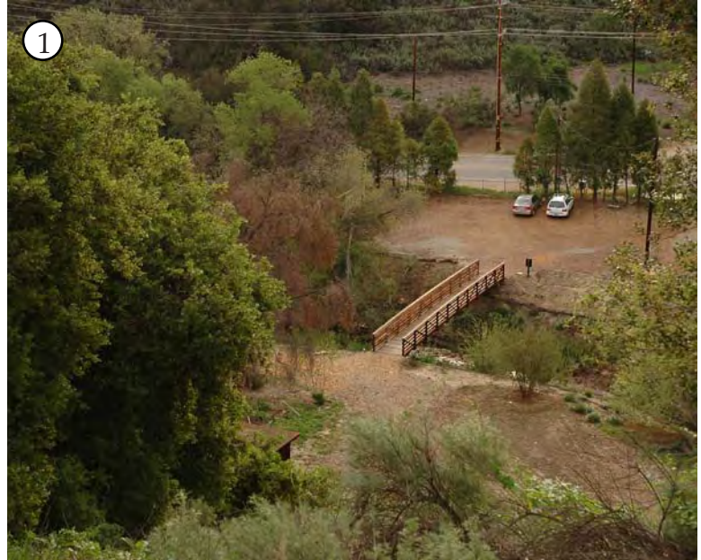
View looking down onto main entry to Headwaters Corner. Visitors park on a mulch pad and cross the newly constructed bridge over the restored reach of Dry Canyon Creek or cross another bridge to the Masson House. Mulholland Highway can be seen in the background.
