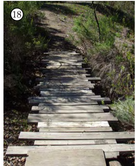
Photo: J.Hall Bridge over historic stream channel connects degraded floodplain terrace and Masson House.
