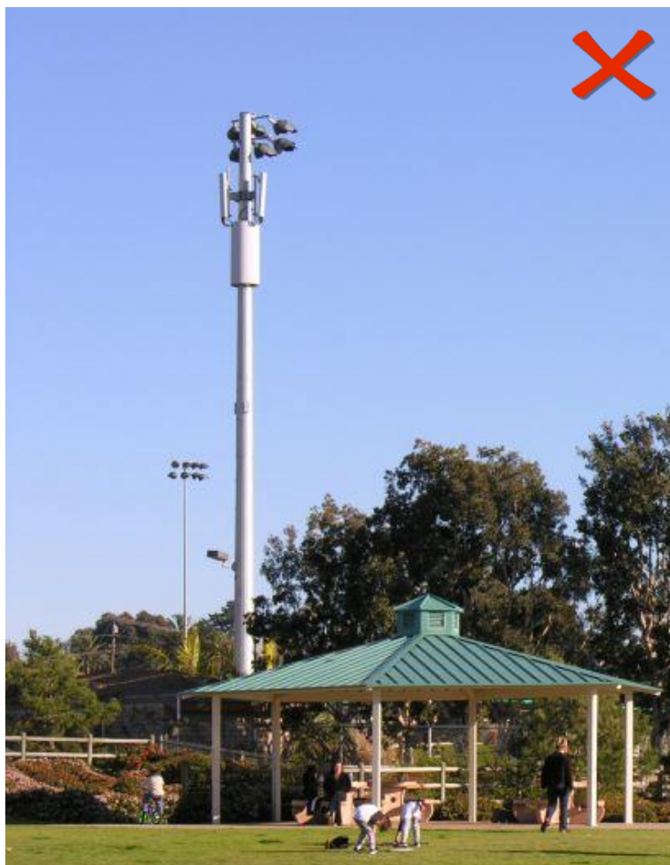
Figure 20: Unsuccessful example at a park outside Calabasas; equipment not fully screened, antennas still visible. Does not meet the classification of a stealth facility not located in the Right-of-Way.
