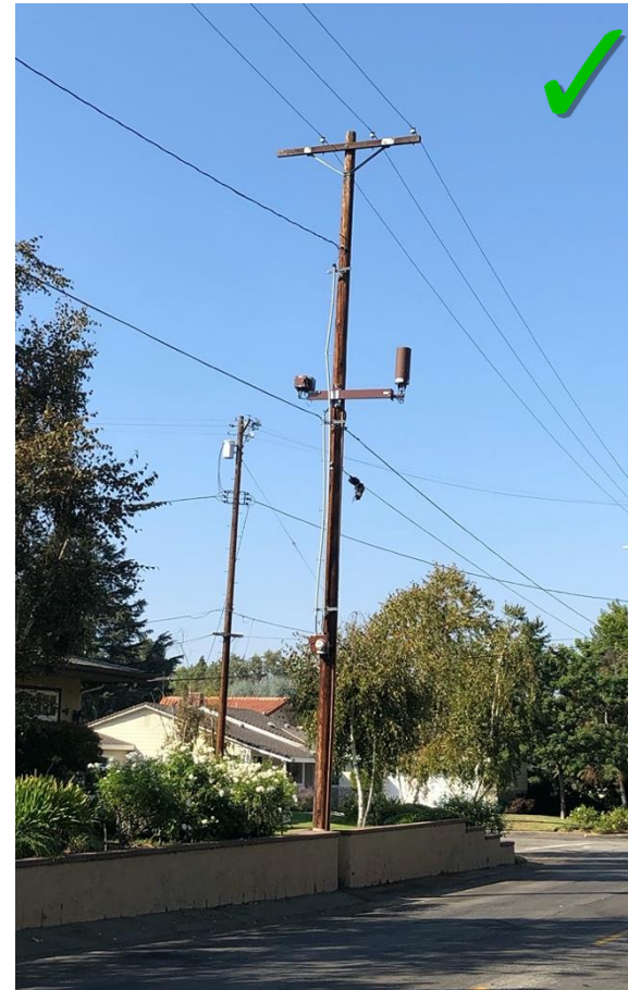
Figure 29: Successful example from outside Calabasas; all equipment and antennas concealed and painted to match pole.
