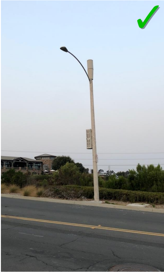
Figure 25: Successful example outside Calabasas; equipment and antennas concealed, no ground mounted equipment.
