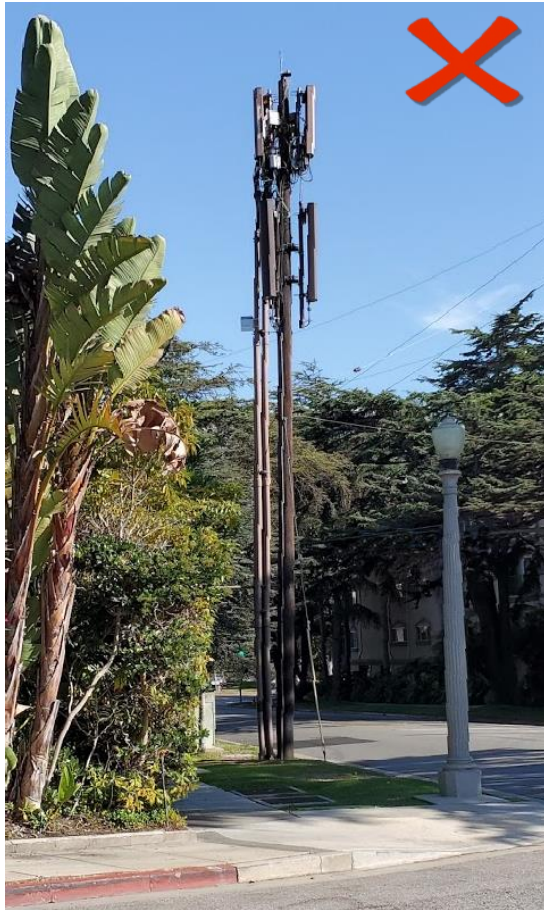
Figure 28: Unsuccessful example from outside Calabasas; equipment/antennas not screened to the maximum extent feasible, visible wiring.
