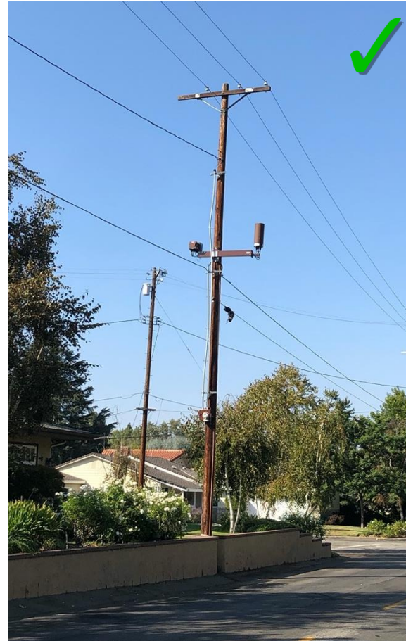
Figure 29: Successful example from outside Calabasas; all equipment and antennas concealed and painted to match pole.
