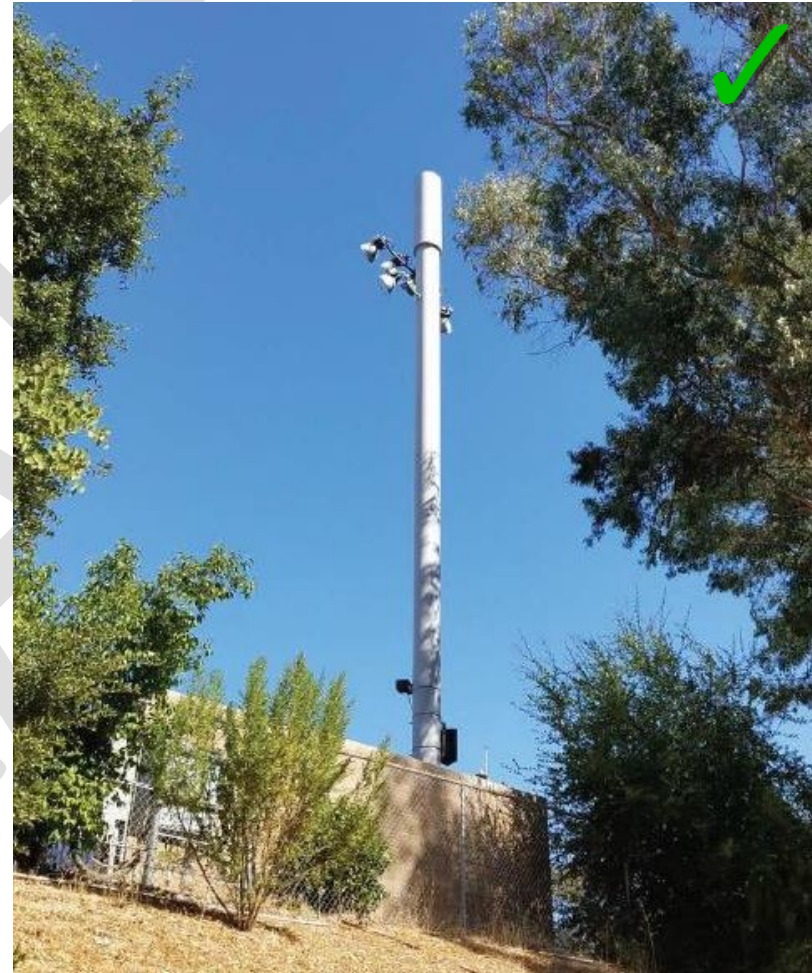
Figure 21: Successful example from facility at Calabasas High School; all equipment screened, and radome camouflaged to match pole.
