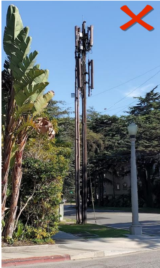
Figure 28: Unsuccessful example from outside Calabasas; equipment/antennas not screened to the maximum extent feasible, visible wiring.
