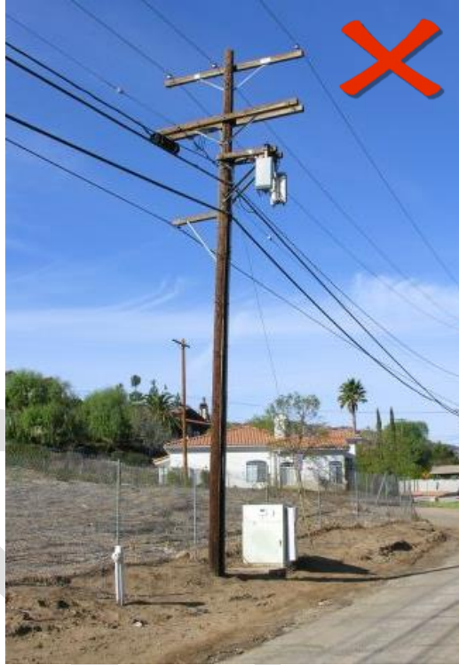
Figure 31: Unsuccessful example outside Calabasas; antennas and ground mounted equipment are not camouflaged through use of paint to match pole.
