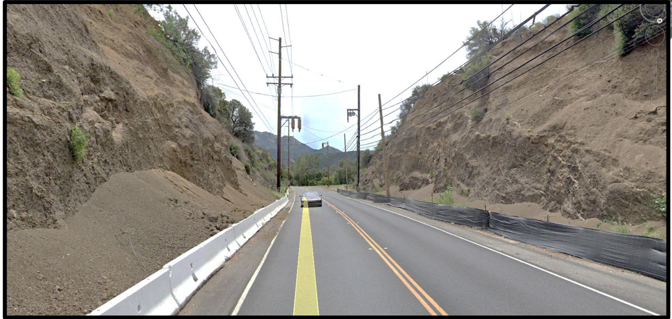
Existing Issue: Hillside Erosion
